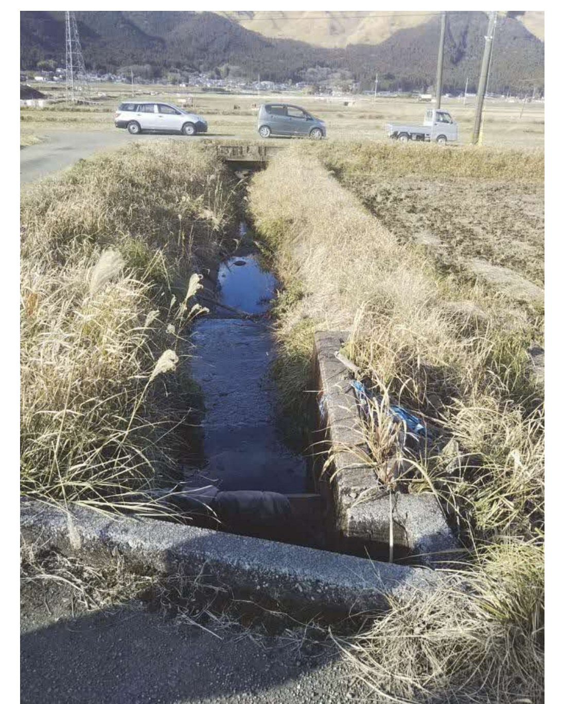
Water canal using ⇒ natural groundwater
